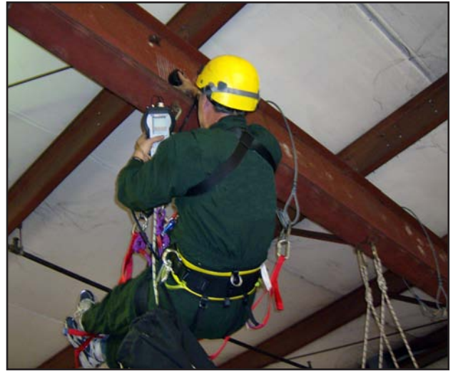
An area of interest was confirmed to be badly corroded after being scanned with the Pocket UT and Z-Scan.
